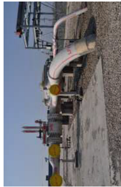
Existing Gas Supply Infrastructure
