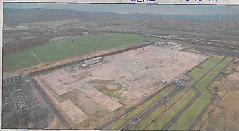
SITE: Sembcorp Utilities UK has revealed plans to build a plant on land previously occupied by the Teesside Power Station
